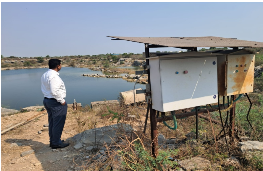
Pump set and Pipe Line installed for supplying Water from Reservoir to Adjacent agricultural fields
